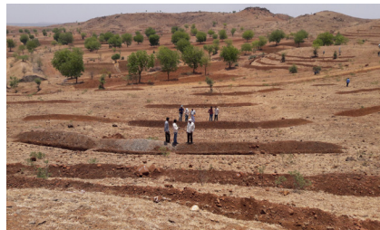
Capacity Building Phase: Watershed structures being created to arrest rain water runoff
